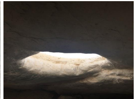
Hullet i taket.
